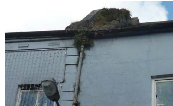
Blocked and leaking cast iron downpipe
