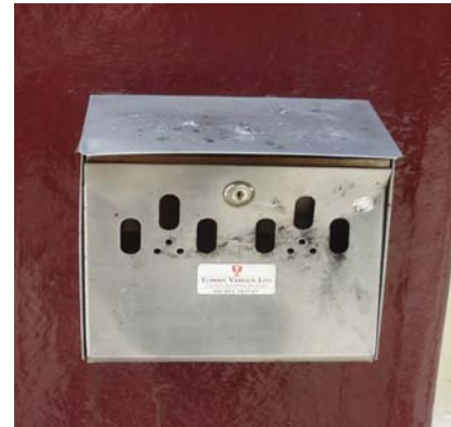
Ash tray fitted to front of historic shop front
