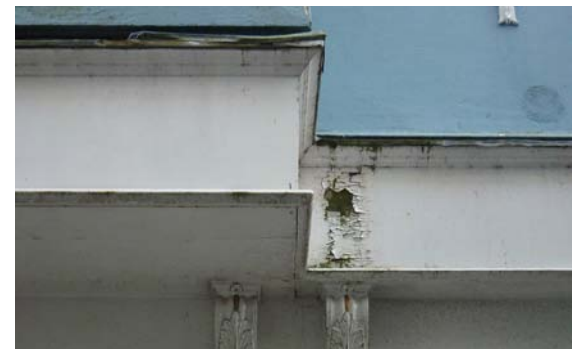
Modern shop front in need of repair & redecoration
