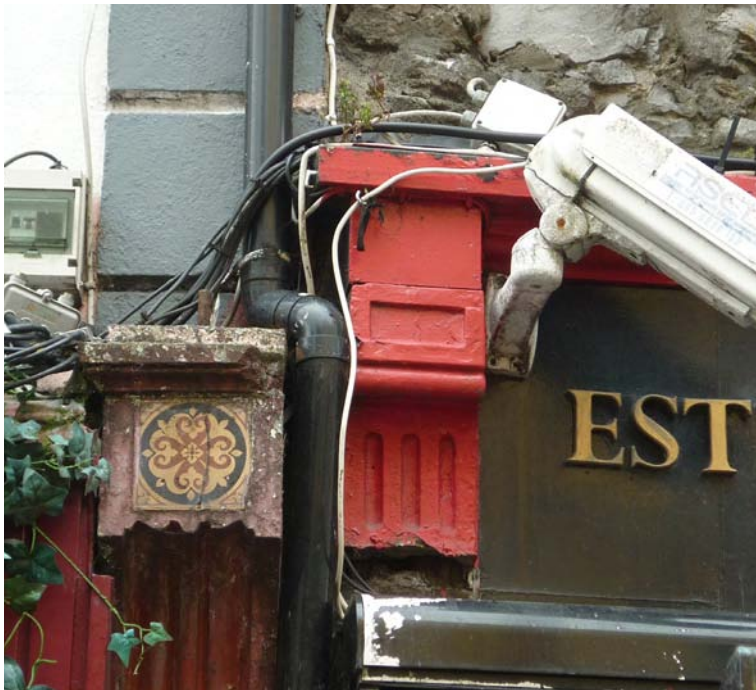
Detail showing poorly coordinated services
